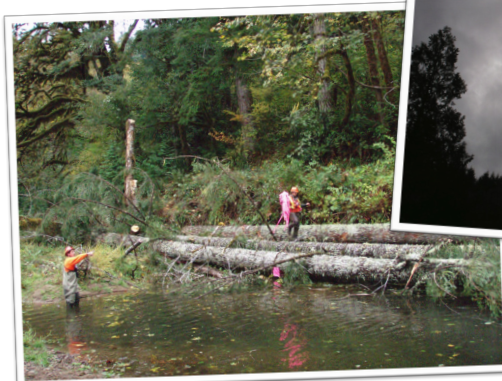
Left: A crew discusses the next placement Right: A log is flown towards a structure site by a Chinook
